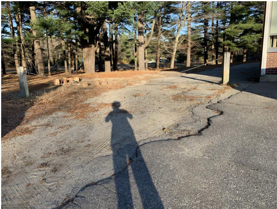
Williams-Cone School termination of NW parking area at northern end of building
