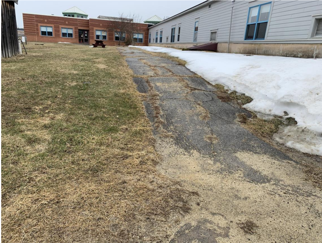
Bowdoinham Community School rear walkway where stairs are needed
