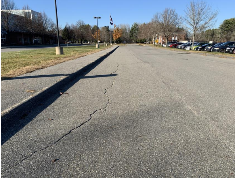
Mt. Ararat Middle School Republic Ave access drive facing north with east parking area on right
