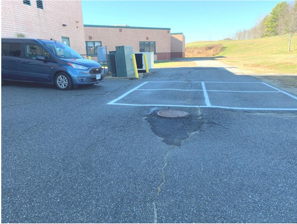
Bowdoin Central School rear service drive/ playground - note heaves
