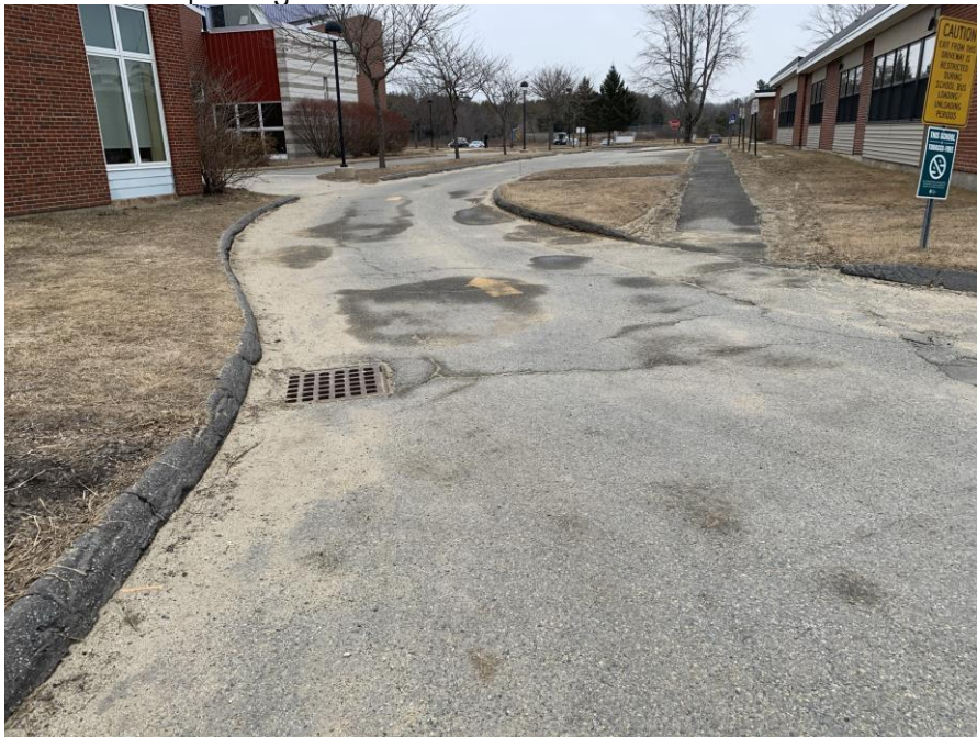
MSAD Office drive connecting parking area #2 to Republic Ave and parking area #2
