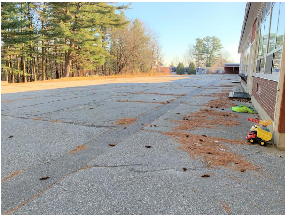
Williams-Cone School paved playground in very poor condition
