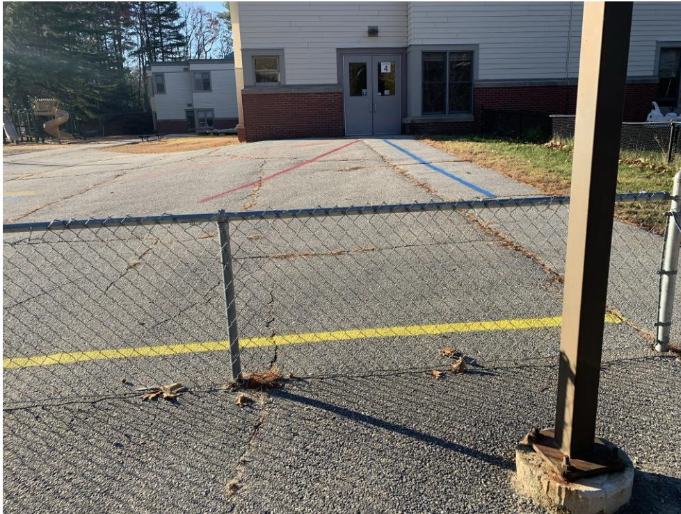
Woodside Elementary School looking at paved playground from end of southern parking area
