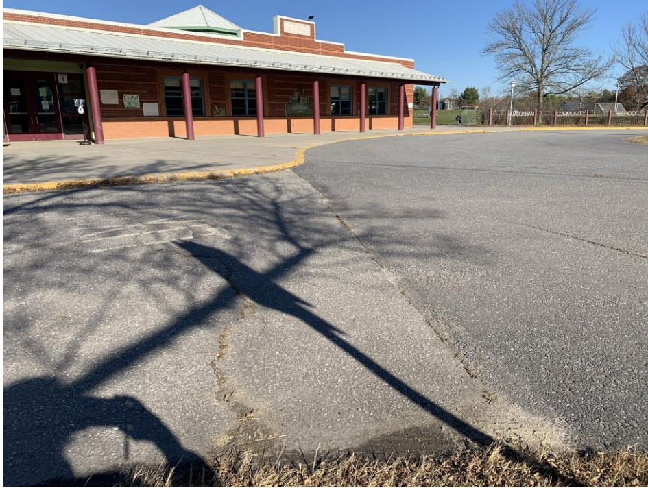
Bowdoinham Community School junction of front walk, bus loop, and main parking area
