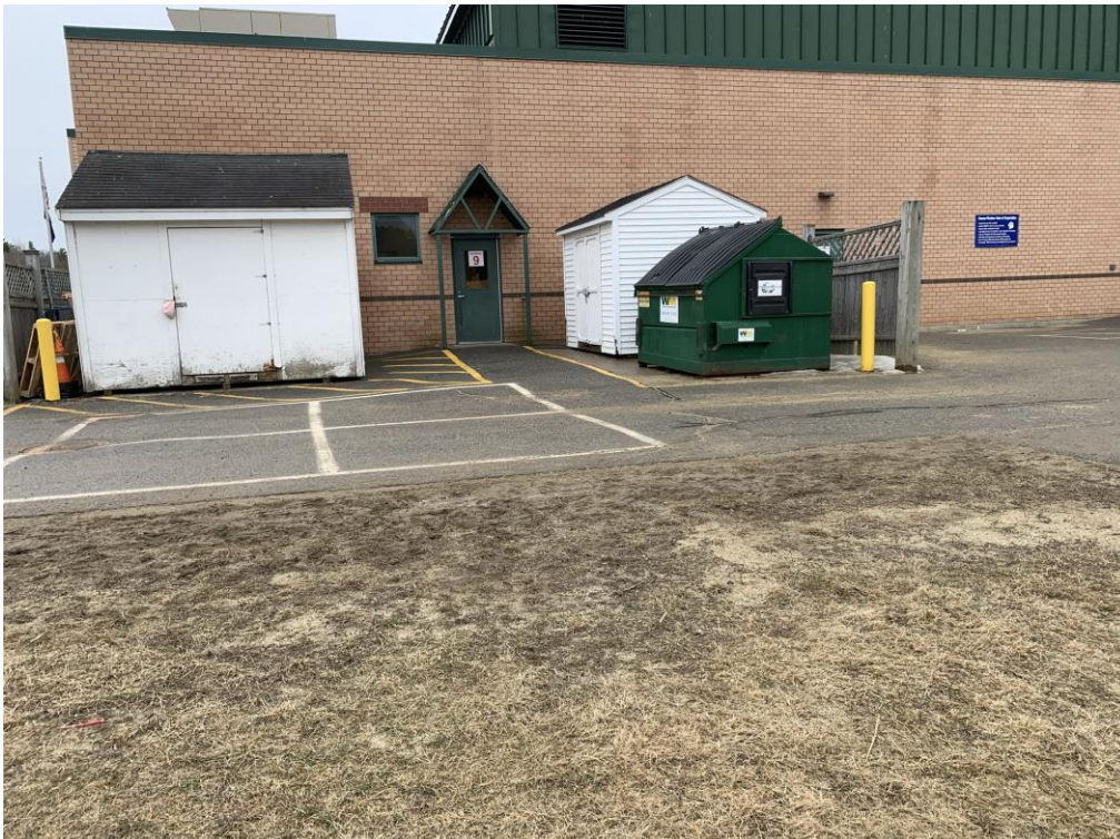
Bowdoin Central School: Deformed pavement/ heaving can be seen near the shed on the left.
