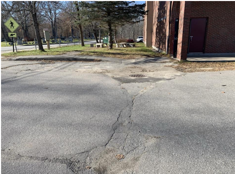
West end of main parking area- note significant pavement deterioration due to ponding at catch basin
