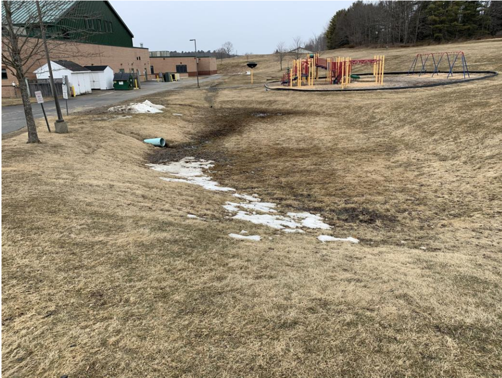
Bowdoin Central School: Poor drainage at rear of school
