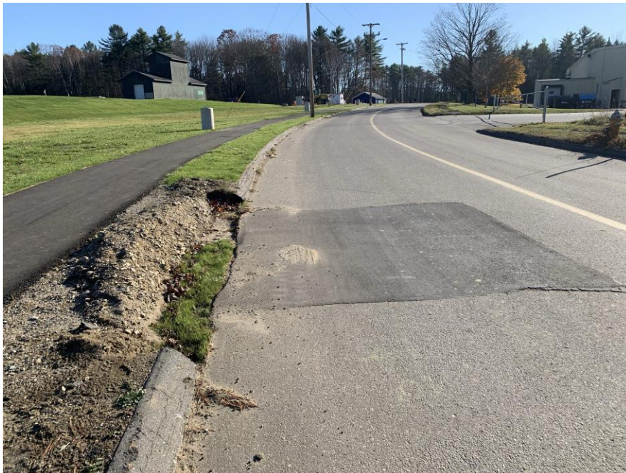
Republic Ave, facing south toward the Aux Parking lot, showing utility patch. Note new sidewalk.
