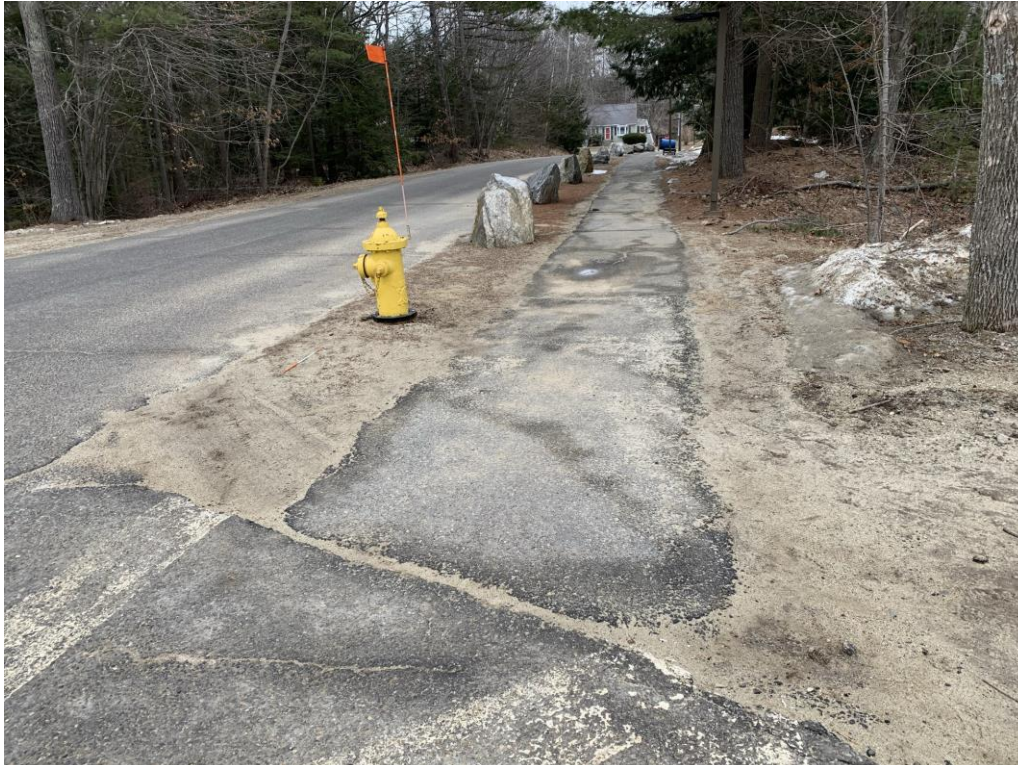
Sidewalk extending from the southern parking area along exit drive out to the Barrows Street
