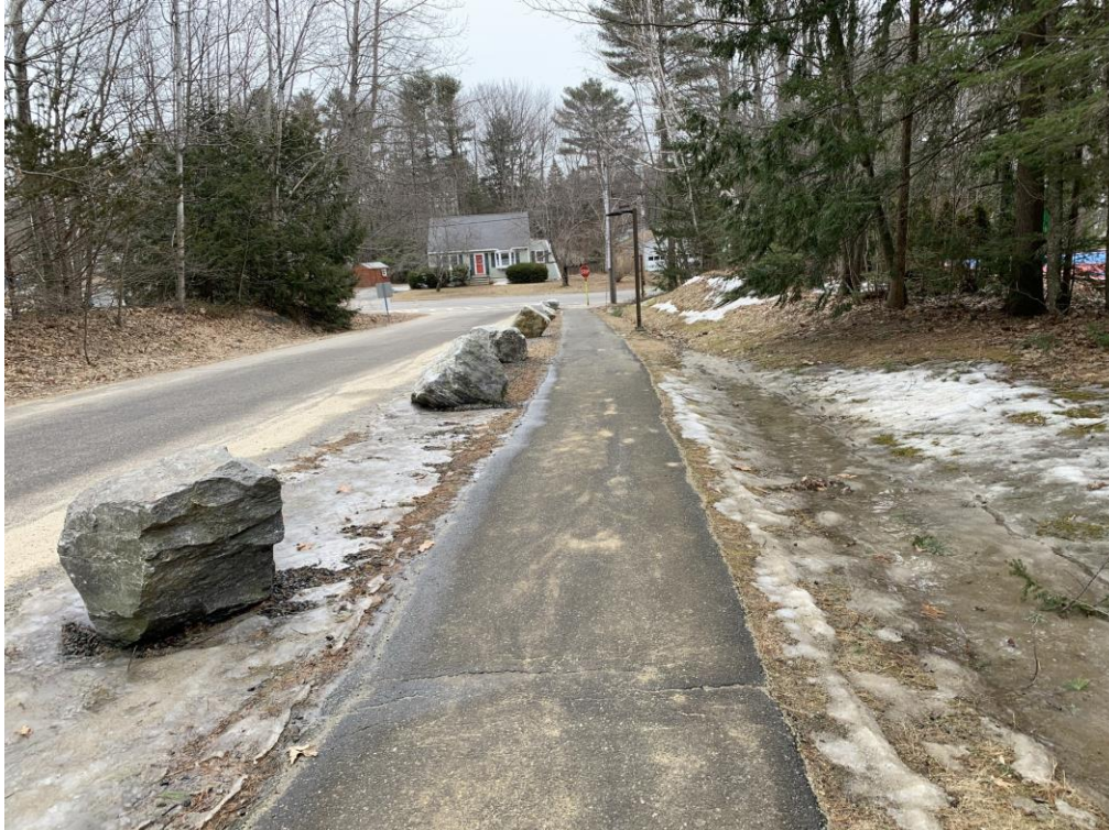
Sidewalk extending from the southeast parking area along exist drive out to the road
