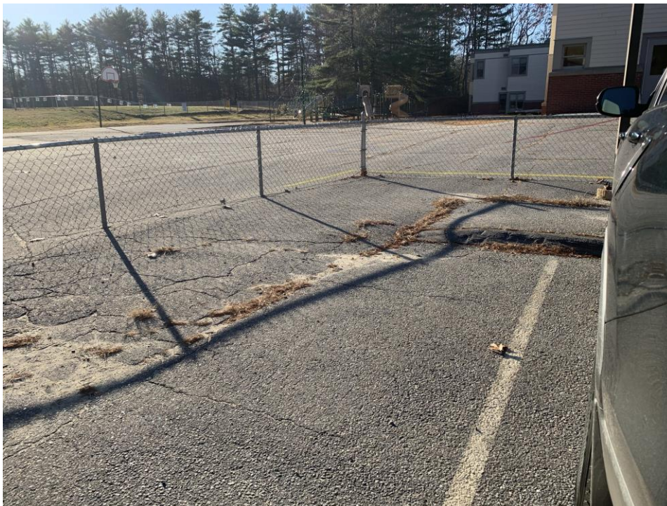
Woodside Elementary School looking at paved playground from end of southern parking area
