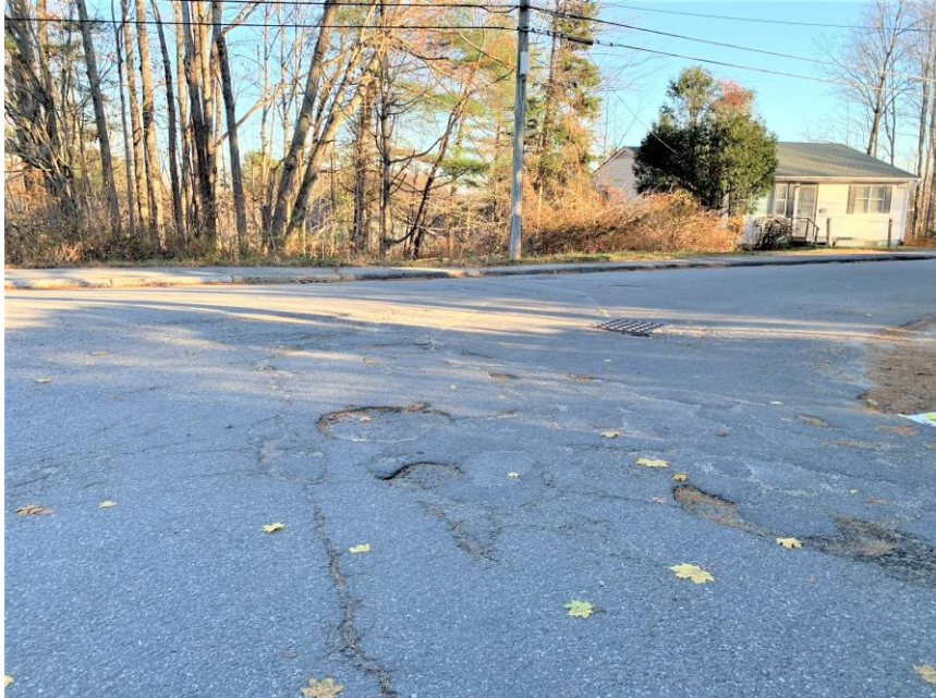
Williams-Cone School main entrance drive at junction with Perkins Street is in poor condition
