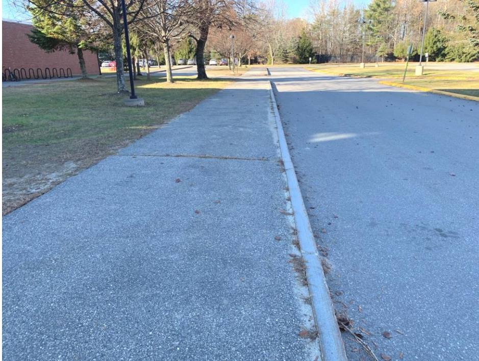
Mt. Ararat Middle School Sidewalk along bus lane looking north toward U-turn
